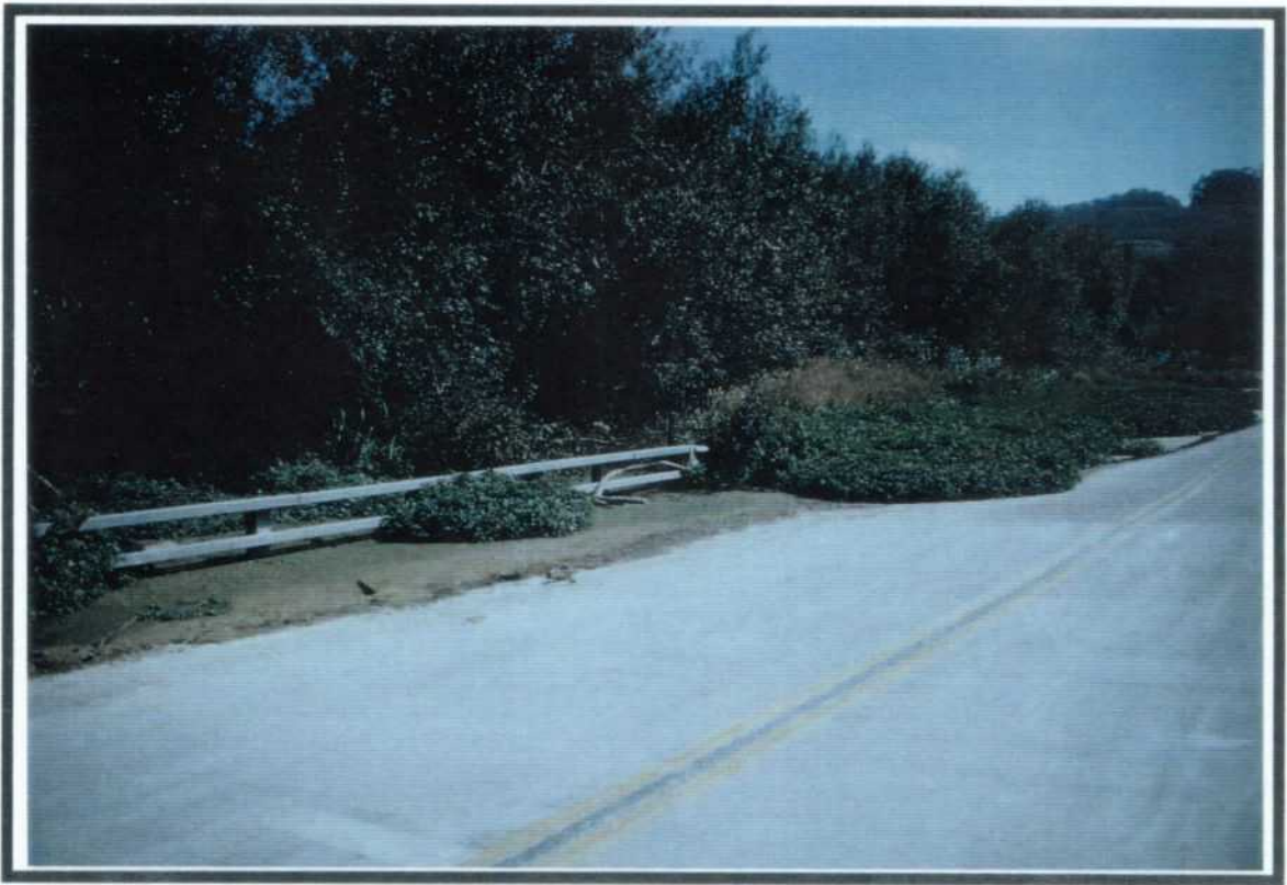
Figure 43. Silt deposition resulting in stream flow changes at Lompoc-Casmalia Road crossing of San Antonio Creek, Vandenberg Air Force Base, California from spring 1995 storms.
